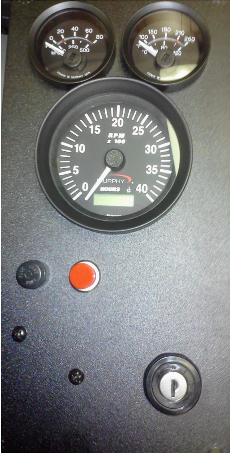
Figure 2: Engine Control Box
